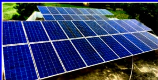
Solar System Setup of 13 kw.
